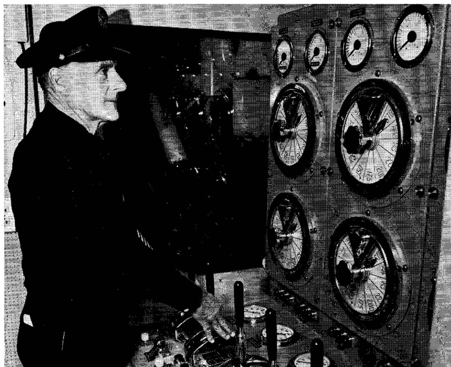
Engineer Sam Le Doux manipulates levers and checks pump rpm's in pump control room just aft of Fire Boat #4's engine room.
